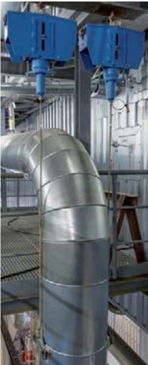
Constant hanger in a coal-fired power station
