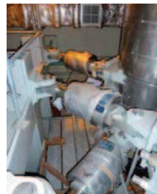
Securing pipe systems with snubbers type 30
